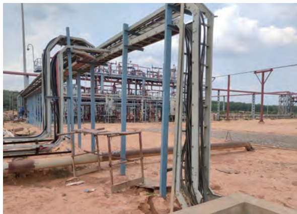
GRP cable ladder at onshore applications
