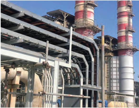
Mesaieed Power Project Qatar
